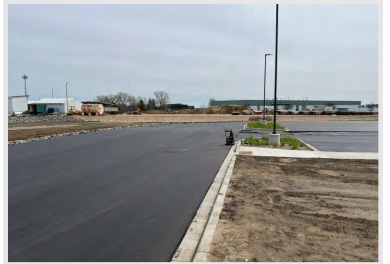
The first half of the parking lot receiving the asphalt topcoat on Friday, April 26 th .
