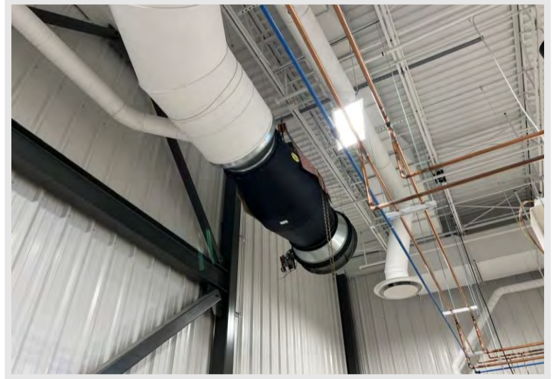
Components of the dust collection system being installed in the Welding & Metal Fab. Lab.
