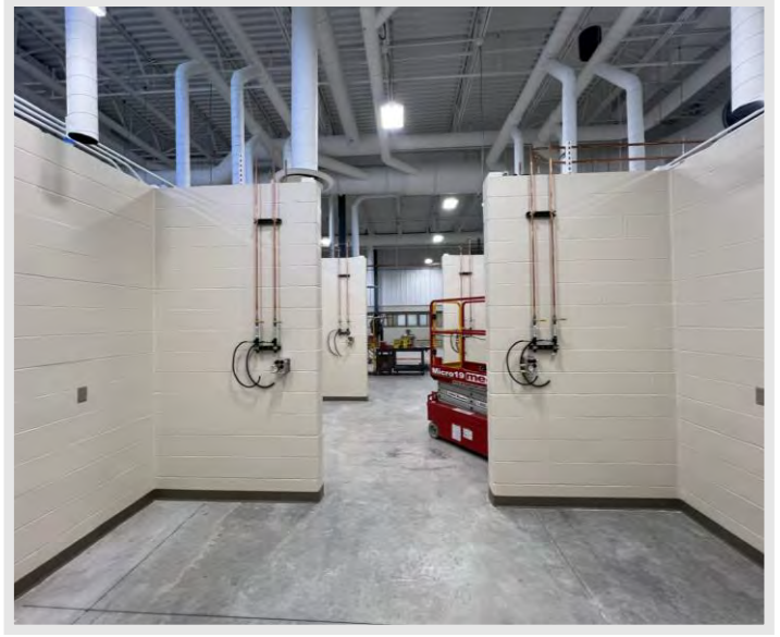
Weld gas piping continues in the Welding Lab and final drops have started to make there way down to mixing valves in each booth.
