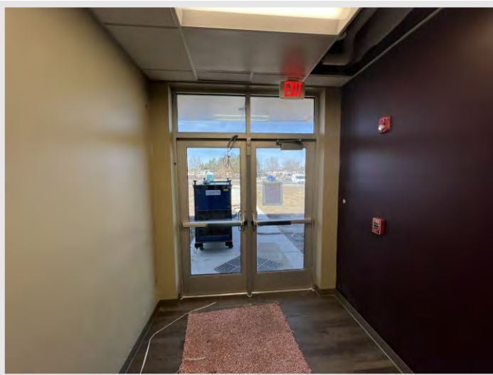
Glazing was installed at exterior storefront doors where heaters were previously routed.
