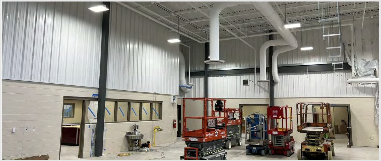
The Welding Lab roof deck is painted, the floor is sealed, and the lights are flipped on!
