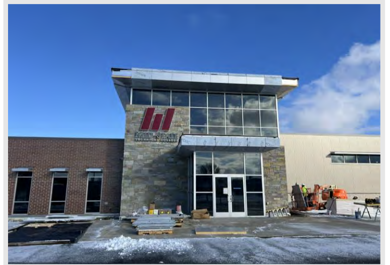
Exterior signage is starting to be installed around the building—above is the main entrance!
