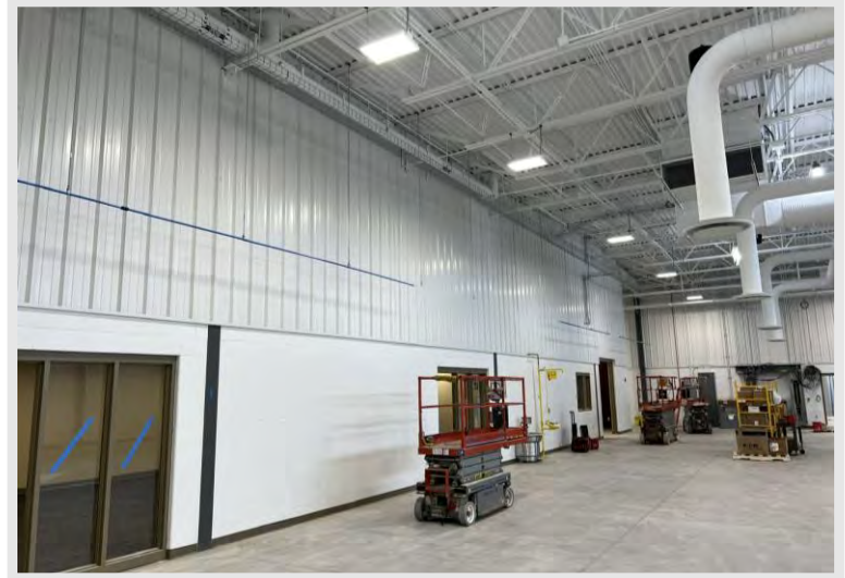
The compressed air piping installation has kicked off in the Machine Tool Lab and will continue in the weeks ahead.
