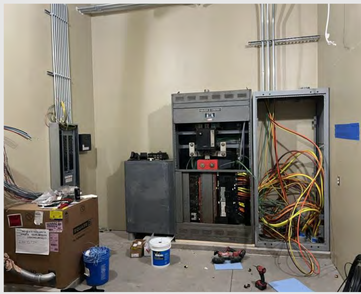
Temporary switchgear was installed on the project to provide temporary power throughout the building.
