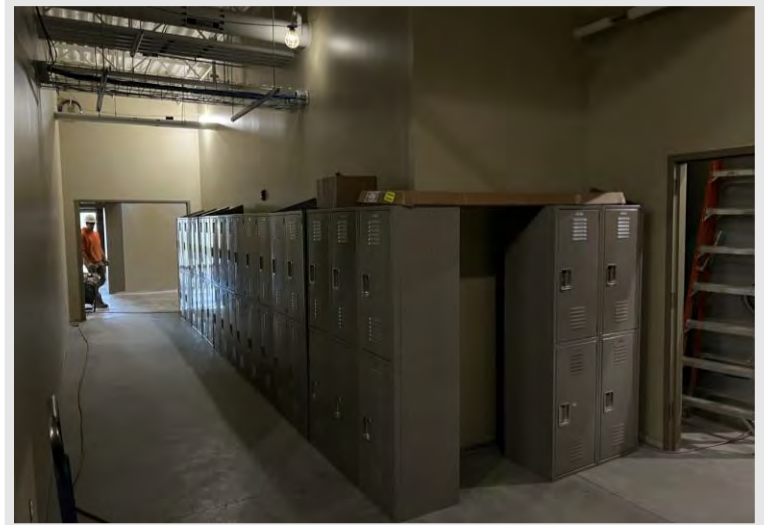
The metal lockers for the project were delivered and will be installed in the various labs in months ahead.
