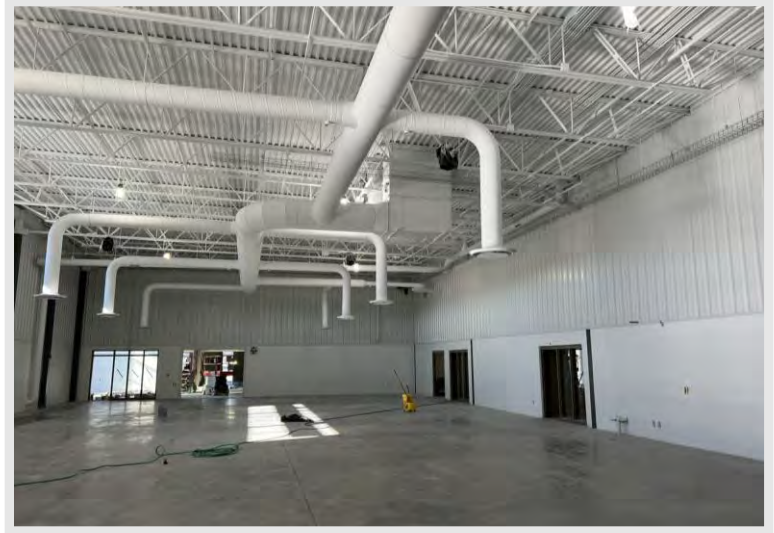
The Machine Tool Lab had the ceiling, and exposed mechanical, electric, plumbing, and fire protection components painted in the last week.
