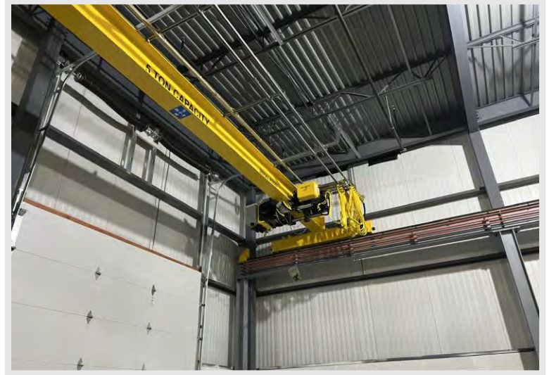
The yellow bridge crane stands out as it has been installed in the Welding and Metal Fab. Lab. It now awaits final connections.
