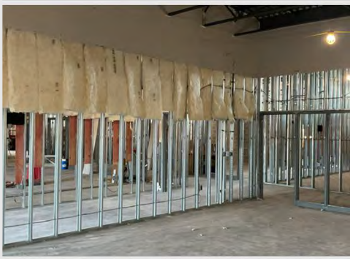
Insulation and drywall has started working from the ceiling down in areas without in-wall mechanical, electrical, and plumbing (MEP) trades.
