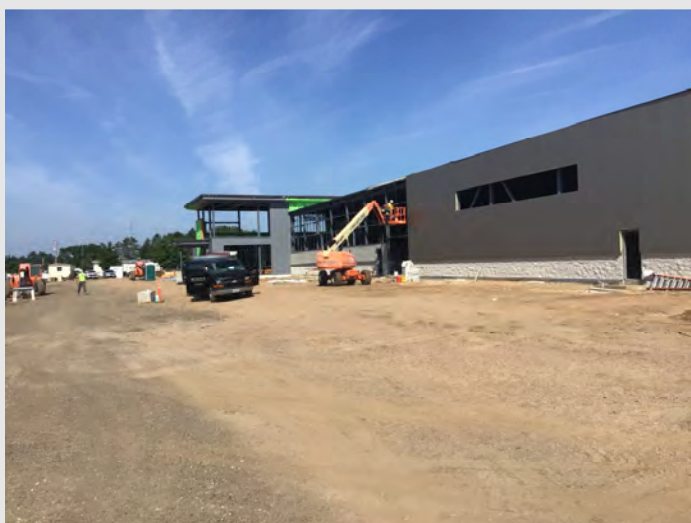
Insulated metal panel continuing its way down the south face of the building.
