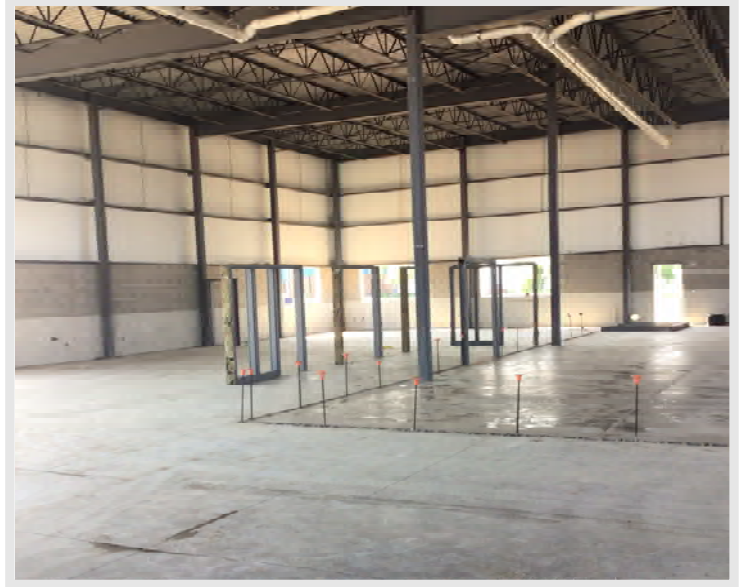
Door frames are being installed ahead of interior metal framing and masonry
