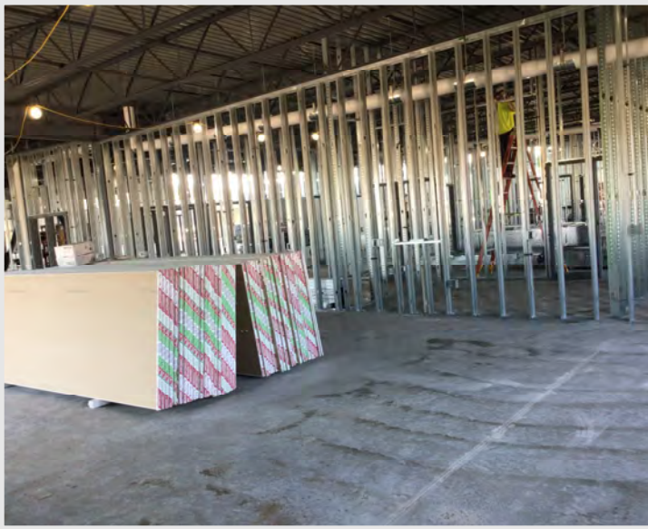
Interior framing has started inside of the building, with our mechanical, electrical, and plumbing contractors working to get their work installed.
