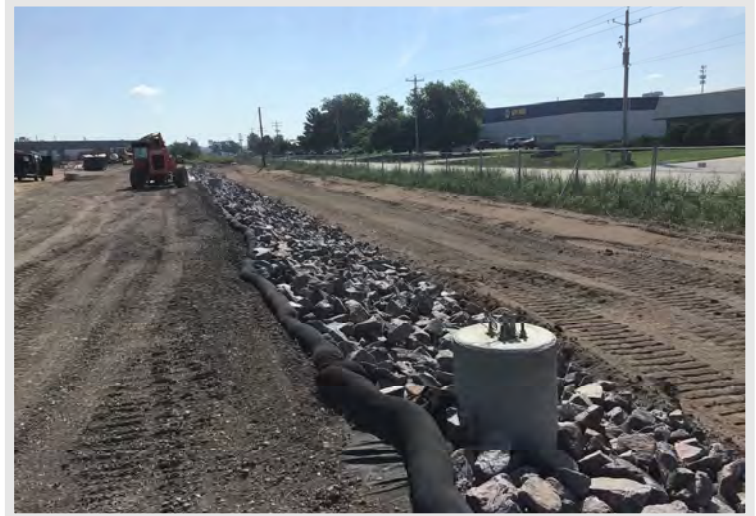
Cosmetic site work has started around the outside of the site with rip rap, and light pole bases being installed
