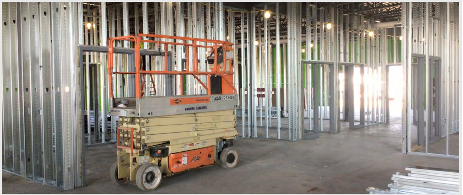
Interior metal framing going up, with the layout of the space starting to come together!
