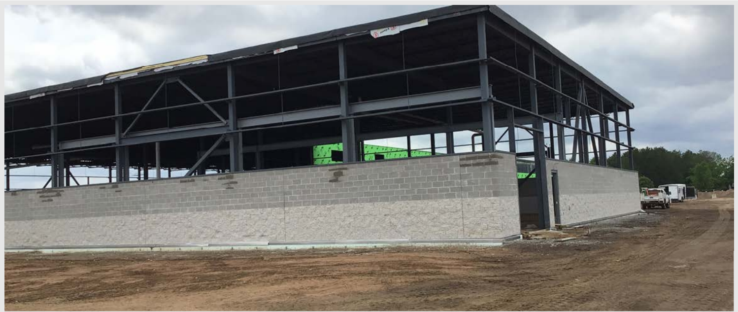
Split face masonry completed on the north end of the building ahead of the insulated metal panel installation.
