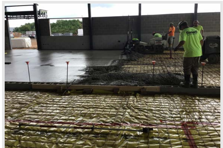
Concrete is being poured, as the first of the interior work is beginning.
