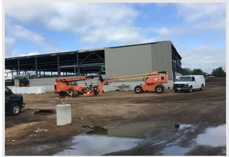
Insulated metal panel is starting to be hung on the East side of the building.
