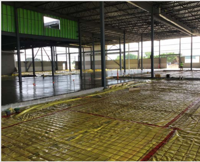
The remainder of the slab on grade is prepped and ready for concrete in the next few days.
