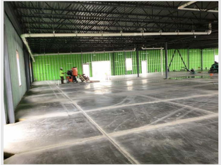
The first section of slab on grade is having control joints cut in to keep concrete cracking in strategic locations.
